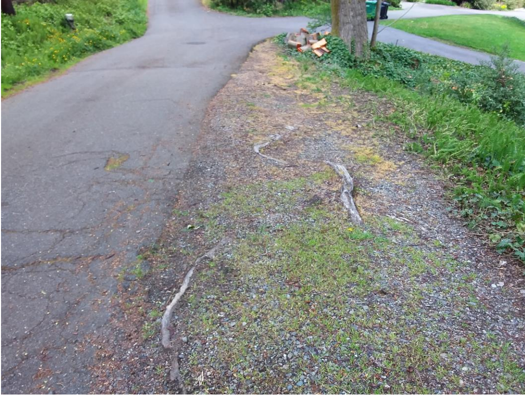
Figure 12. Looking NE down 72 nd and showing surface roots from the #3 and #4 trees in the parking strip. Note the cracking in the asphalt indicative of root pressure.
