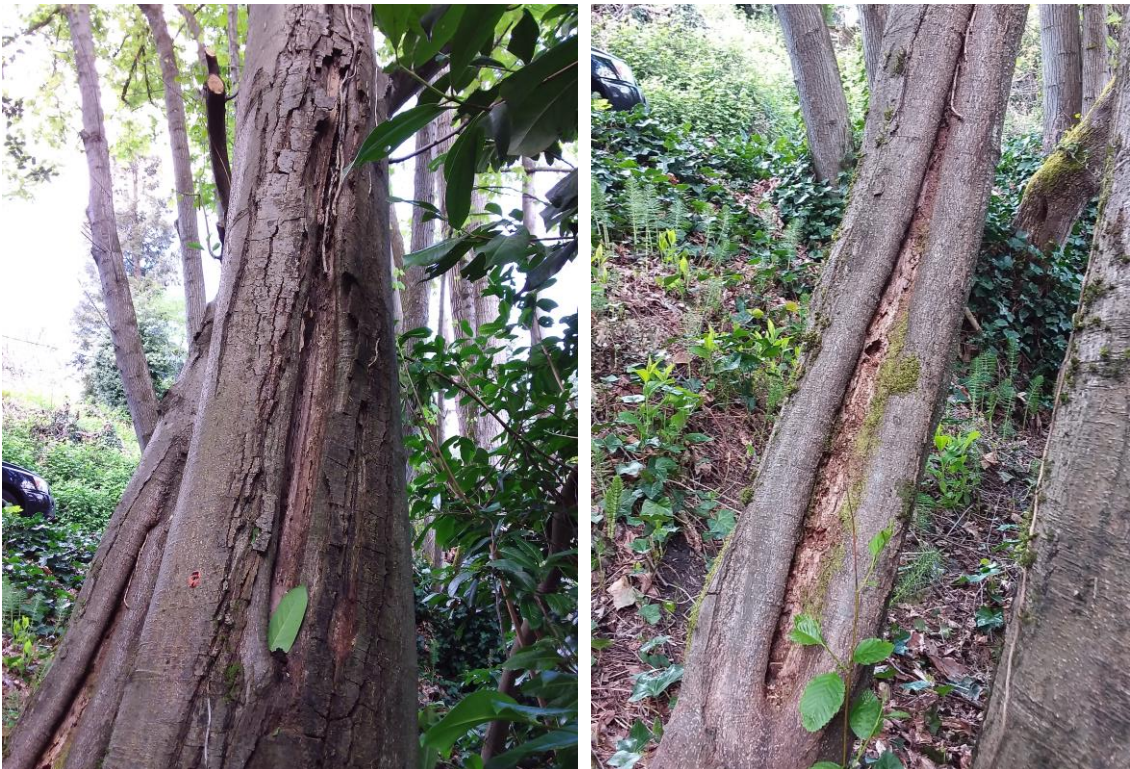
Figures 15 and 16. The main and smaller trunks of the #7 alder showing the advanced decay running up the column of each.
